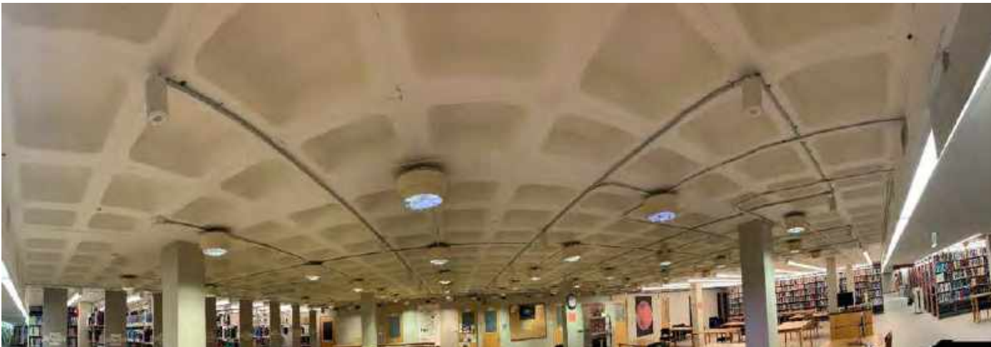
Low floor to floor heights (8'), waffle slab construction, no daylight penetration, no fire suppression system (sprinklers), antiquated fire alarm system
