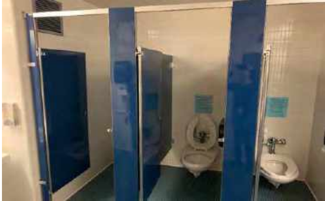
Non accessible restroom entries, toilets, and fixtures; accessible restrooms located on only half of the existing floors.
